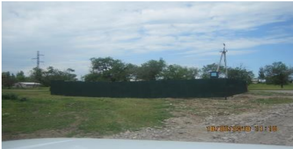
Figure 25 Restored well to supply the plant with water
