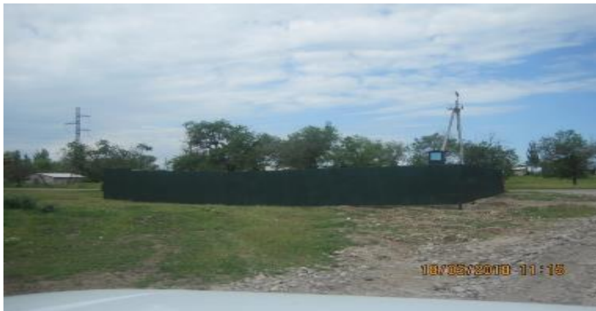
Figure 38 Restored well to supply the plant with water
