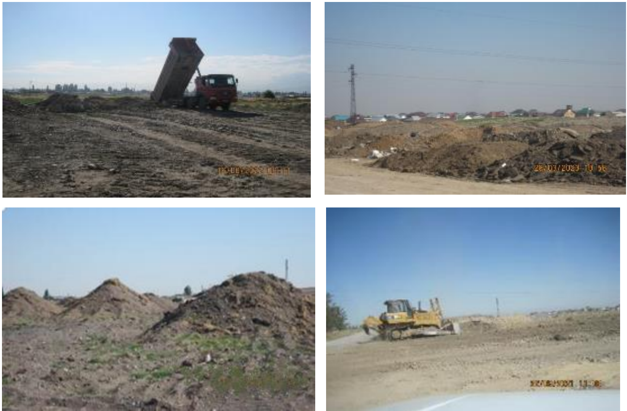
Figure 46. Storage of unsuitable soil for further use in the villages of Voенno-Antonovka
